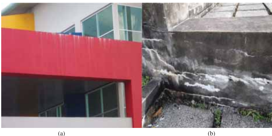
Figure 1: Efflorescence formation on concrete structures.
