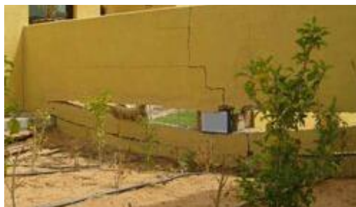
Figure 1. Failure of structures resting on Calcareous soils
