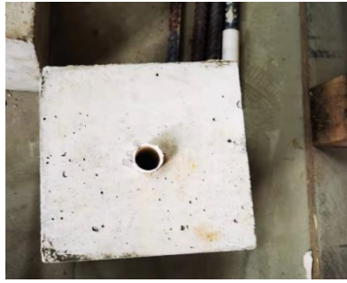
(1) Pull-out damage of rebar
