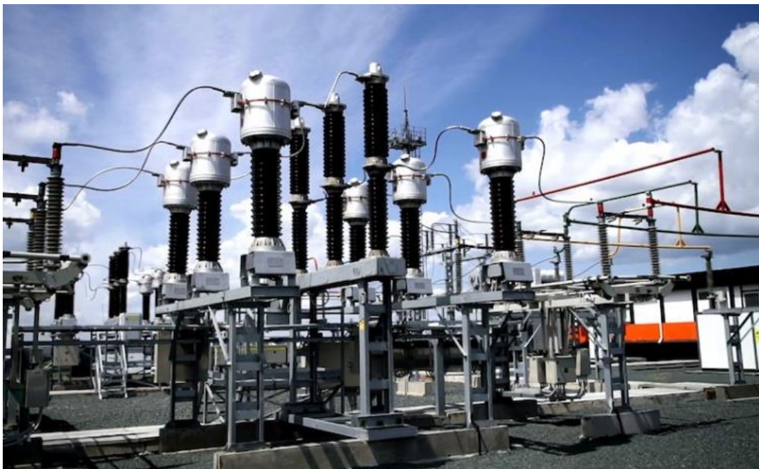
Figure 2. Nigeria's power grid project
