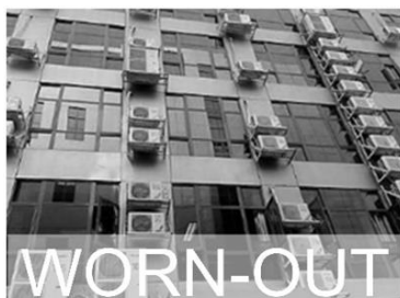
Figure 6. Non-uniform outdoor AC unit arrangement
