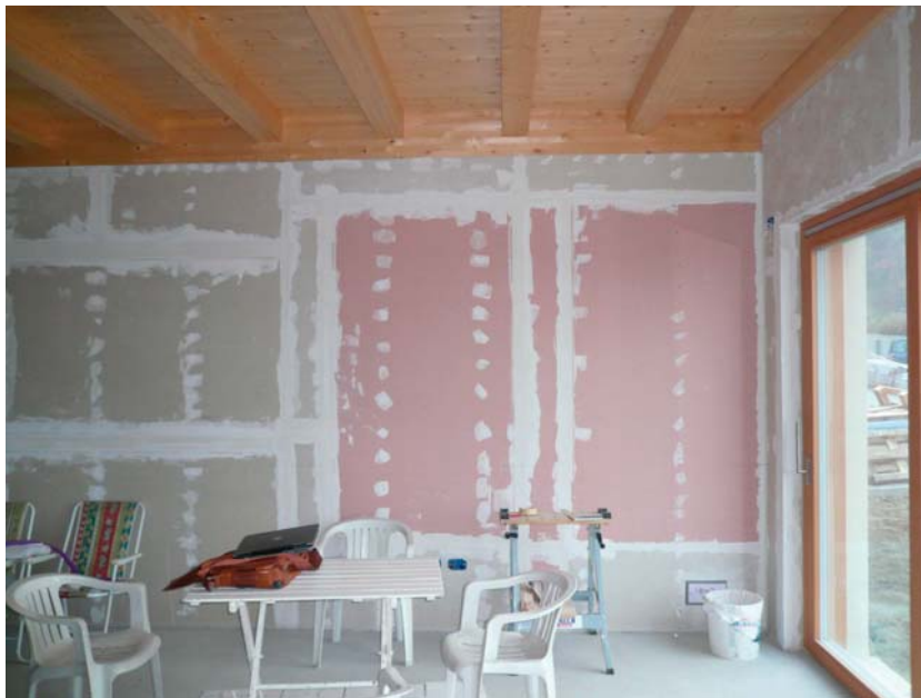
Figure 14: Preparation of radiant wall panels in Micronal PCM (Phase Change Material). The panels contribute to avoid overheating during summer, holding temperature between 22 and 23°C.
