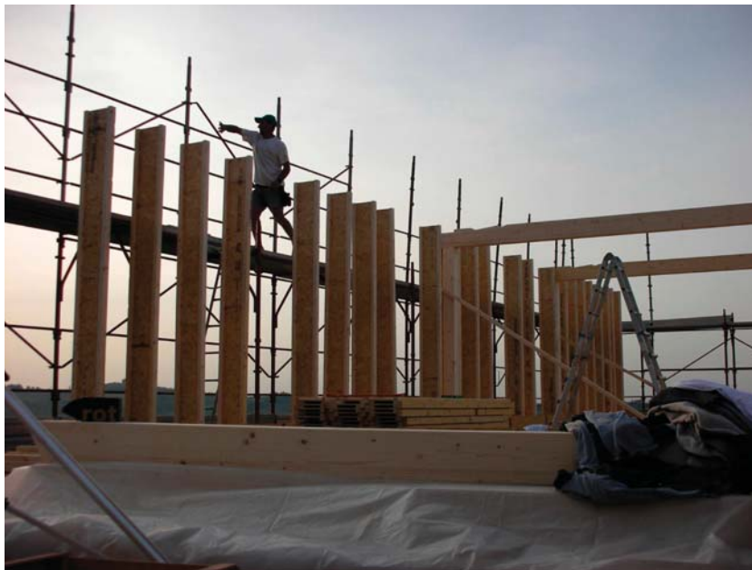
Figure 11: The wooden structure erected on the reinforced concrete basement. The concrete portions were built in three months. The upper wooden structure was built in two weeks.
