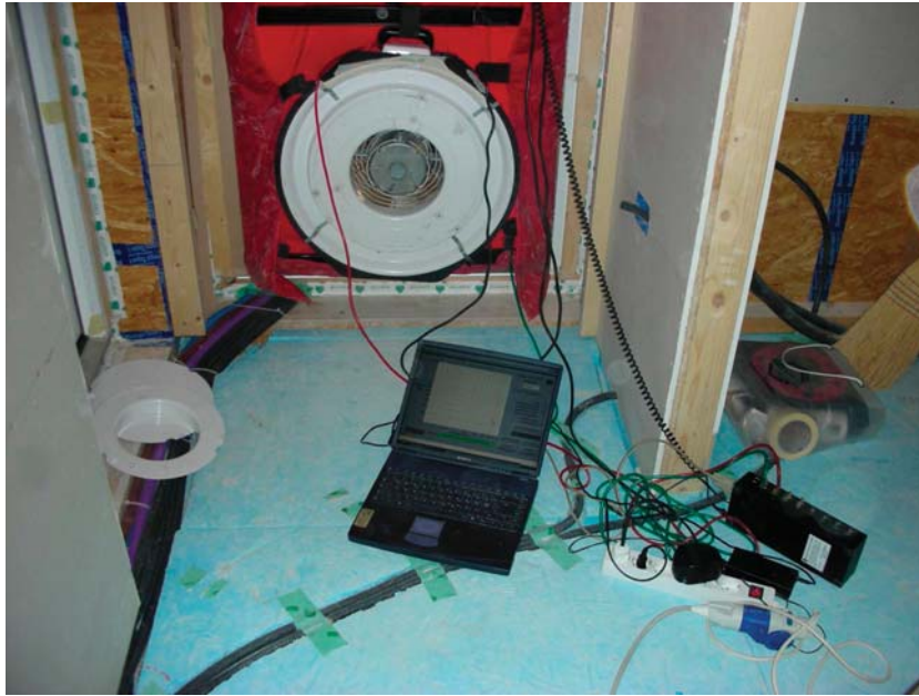
Figure 15: Blower door test. It is a diagnostic tool designed to measure the air-tightness of buildings and to help locate air leakage sites.
