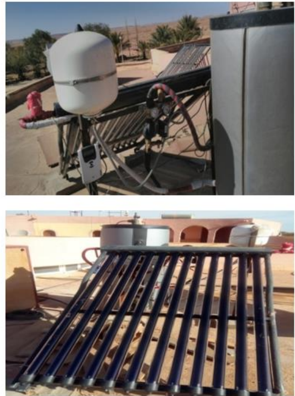
Figure 1. The product IMEXSol 200L installed in Ghardaia region
