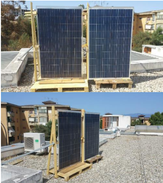
Figure 7. Installed PV panels to carry out producibility measurements in a vertical plane
