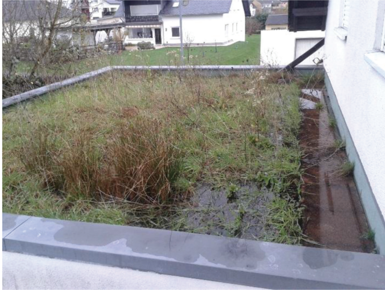
Figure 3: Green roof after loading with nearly 31 mm of precipitation over about 3 days (in the right background is the connecting pipe from the pitched roof)
