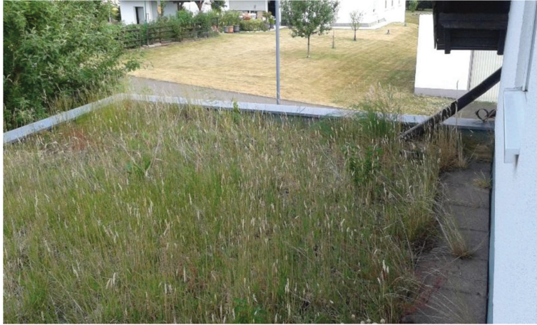
Figure 5: Condition of the green roof on 23 June 2017 after a long rain-scarce period. Compare its colour with that of the lawn in the background (on the right side is the connecting pipe from the pitched roof)
