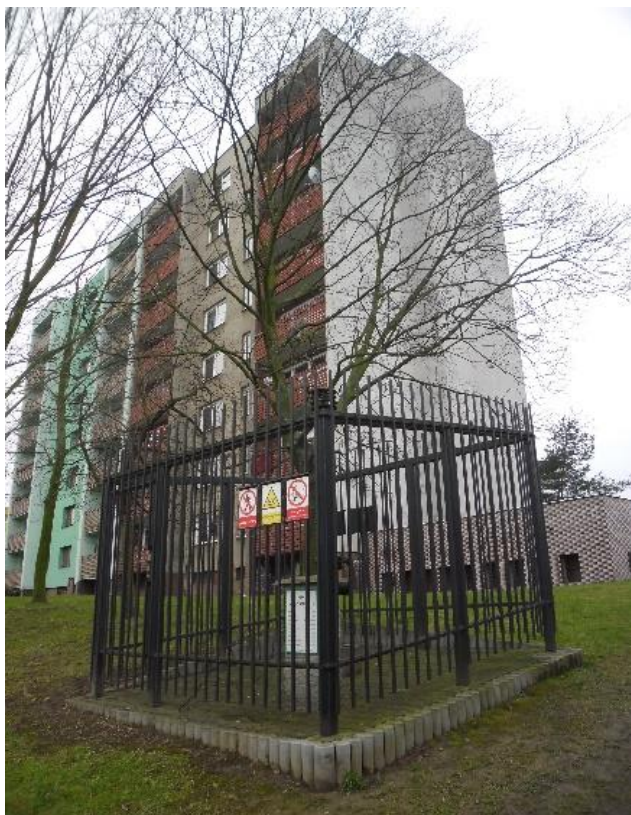
Figure 6. Protection of a panel house at Ostrava - Muglinov by means of gas drainage borehole
