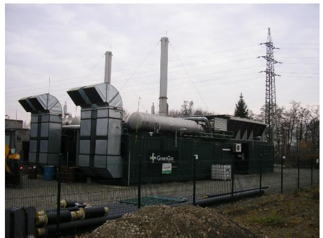
Figure 2. Cogeneration unit from the former František Mine
