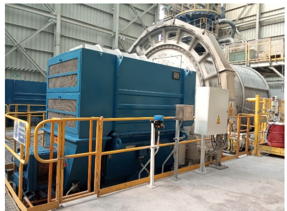
Figure 1. A 2250 kW electric motor driving a ball mill in a concentrator plant
