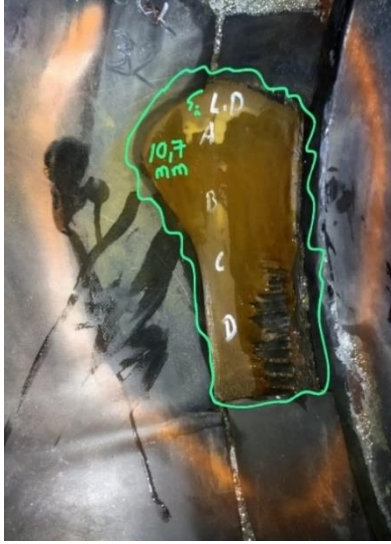
Figure 6. Field Inspection and In-Situ Wear Evidence
