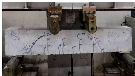
Figure 13. The patterns of cracks for the beam B3
