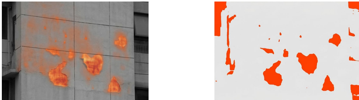
Figure 7. Multi-modal registration fusion and intelligent segmentation results of building exterior wall debonding defects
