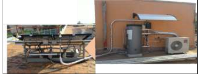
Figure 4. PVT plant at the University of Catania [23]
