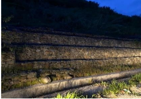
Figure 3. Land protection wall on the slope area on national crossroad, Solok Regency
