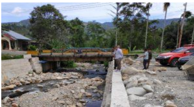
Figure 4. Kapalo Koto River Normalization Project in Lembah Gumanti Area, Solok Regency (Source: Suara Independent News, 2021)
