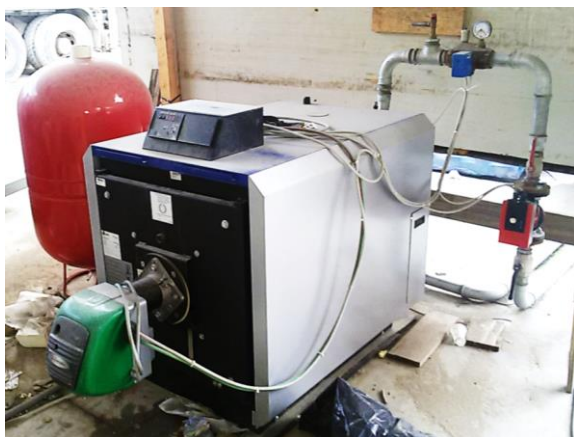
Figure 11. Boiler fueled by LPG for heating the water in the test phase
