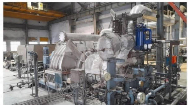
Figure 2. Steam turbine setup in cogeneration power plant
