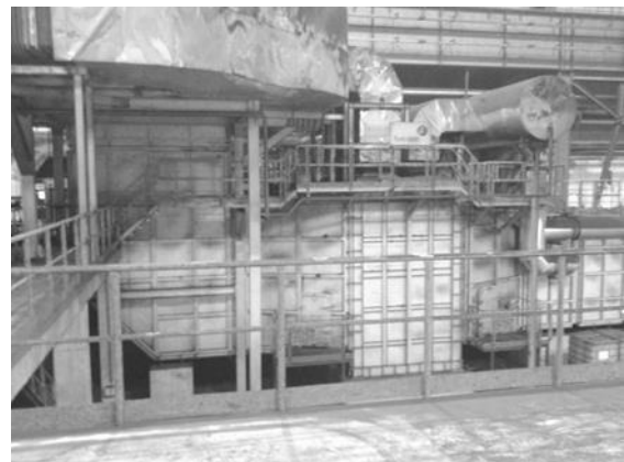
Figure 1. View of an industrial recuperator in a steelworks
